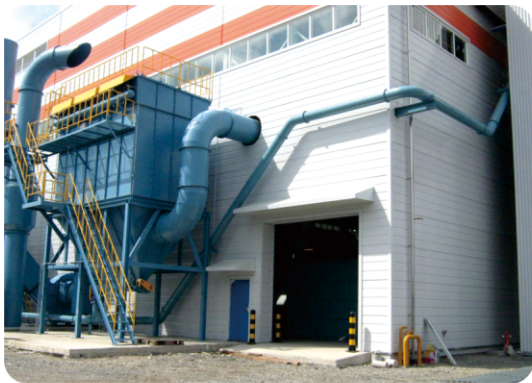
Collecting Dust from each Dust Collecting points using by Suction Pipe Lines.
