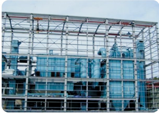
Sand Plant System (150 ton/HR)
