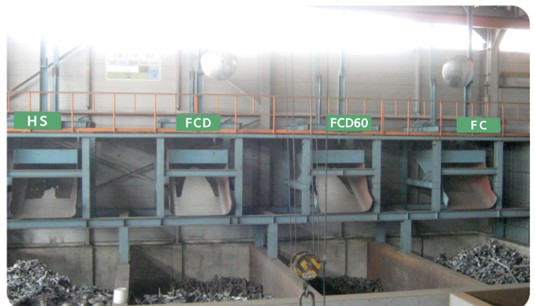
Unloading Bunkear at Electric F. C. E. S Area
