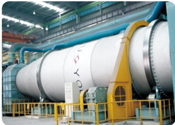
Cooling Drum & Casting Transport System
