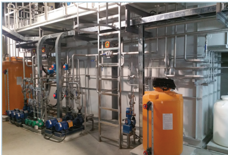
▲ Sewage Water Treatment Package
