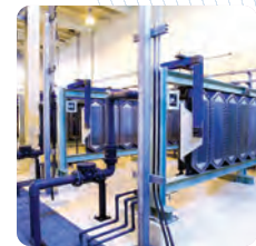
Seawater Electro-Hypochlorination System
