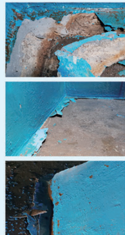
Epoxy coating has also many problem
