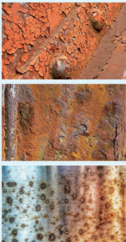
Steel must rust
